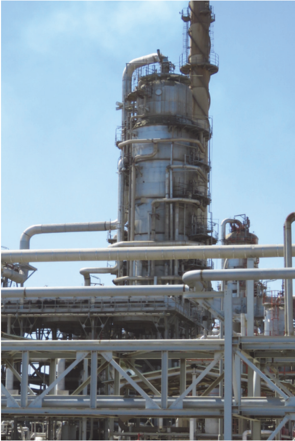
Fig. 2. Phase 3 Abadan Oil Refinery Co
