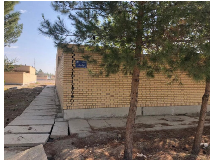
Fig. 3. Land subsidence in one of the regions in Esfahan (Source: Mehrnews)
